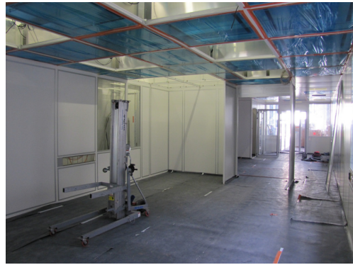
Figure 4: View inside of the clean room (same direction as in Fig. 3), from the ISO 4 area facing towards the ISO 6 and the air-lock area: The double floor is completed, while the installation of the filter-fan units, plumbing and electric installations is ongoing.
