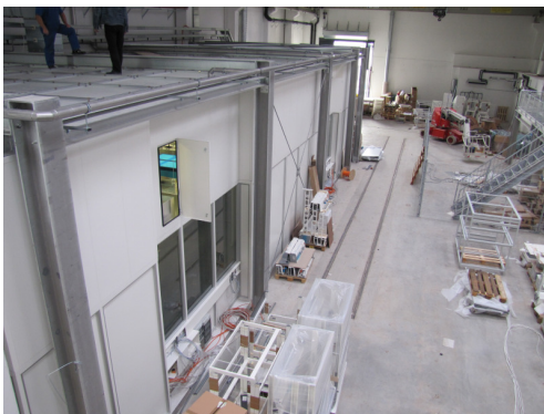
Figure 3: Exterior top- and sideview of the clean room: The outer casing is complete, while the installations inside are ongoing (see Fig. 4).
