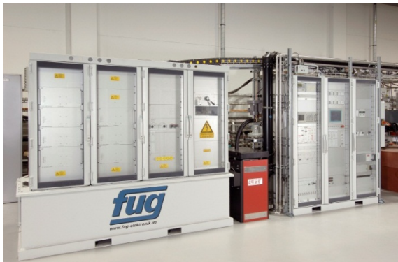
Figure 3: The 80 kW IOT based transmitter used at the MLS. This transmitter is used as prototype for the klystron-based 270 kW transmitters for the injector cavities at BERLinPro.
