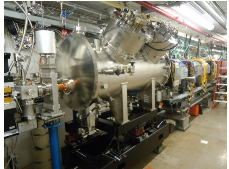
SCU0 installed in the APS storage ring in Dec, 2012.
