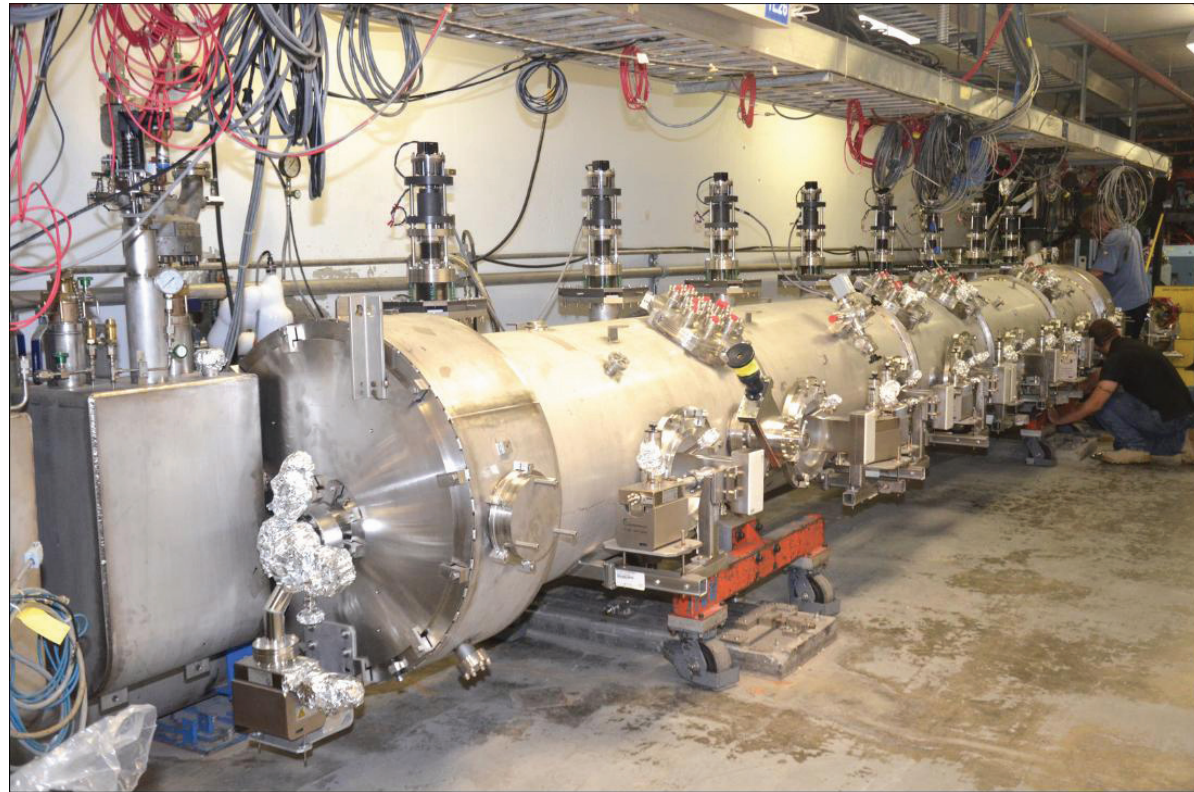
Final C100 installed in linac
