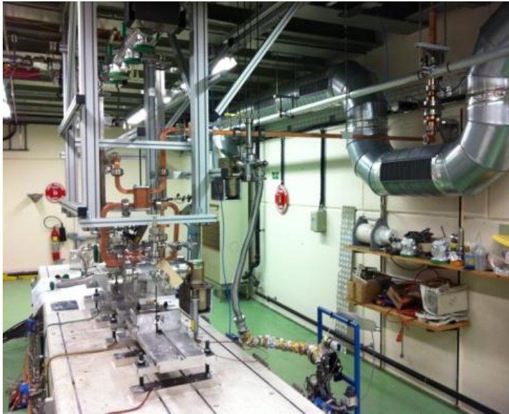
XBOX1 at CERN operational with SLAC klystron
