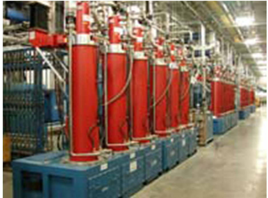
Klystron gallery 550 kW 805 MHz
