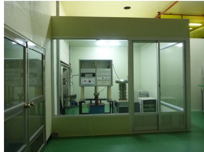
[New Control room(Tunnel)]
