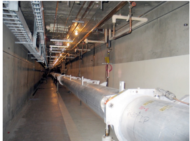
Figure 6: Sector 20 after the accelerator systems were removed. The tunnel is ready for the FACET magnets to be installed.
