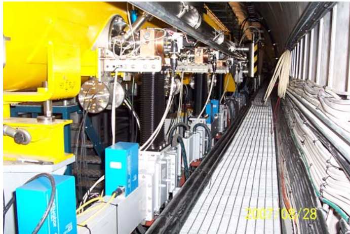
Waveguide distribution for ACC6 with phaseshifters integrated into shunt tees in FLASH tunnel
