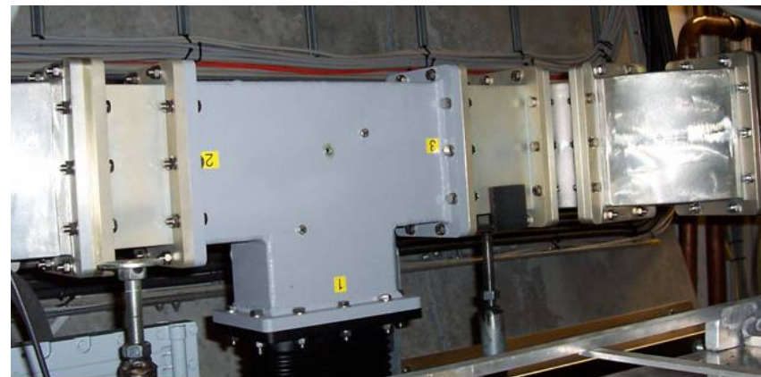
2.4dB asymmetric shunt tee to split RF power between ACC5 and ACC6 in FLASH tunnel
