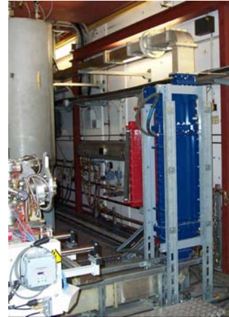
5MW four-port circulator installed in the tunnel before FLASH gun
