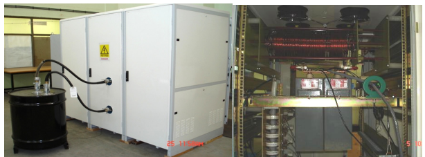
Figure 4: (left) resistive load in oil tank (@110kv) connected to modulator; (right) bouncer circuit elements pictures at RRCAT
