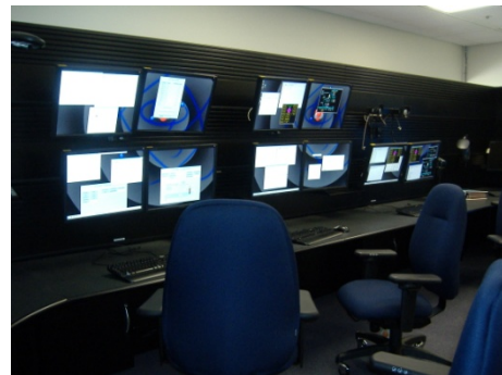
Figure 2: NML Control Room.
