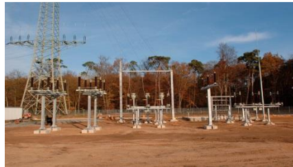
Power grid connection
