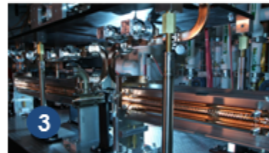
X-Ban RF deflector @ LCLS
