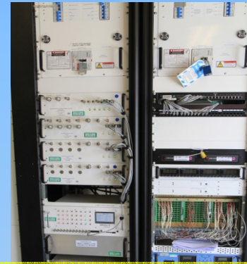
Controls: PAC, PADS, MKSU
