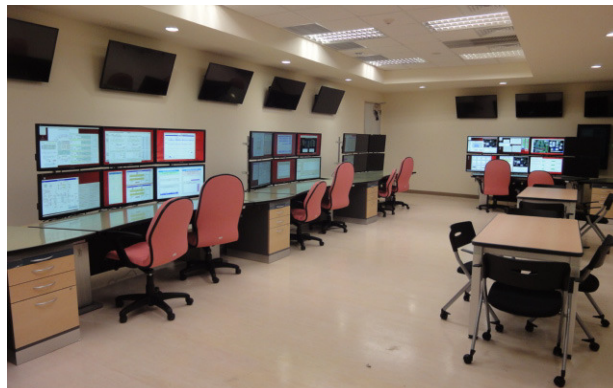
Figure 1: Console in the TPS control room includes multiple LCD screens and ready for use.
