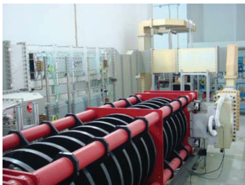
Figure 3: CPHS RF power system.
