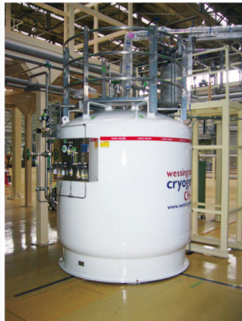
3000L liquefied helium storage vessel
