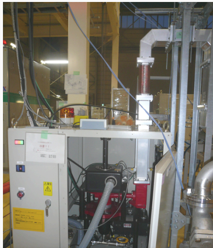
30kW CW IOT for main SCC
