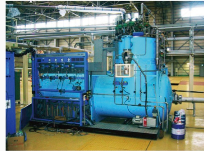
TCF200 helium liquefier/refrigerator
