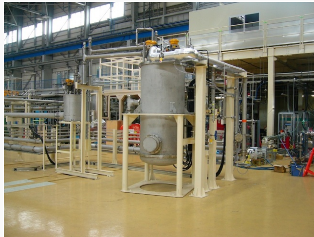
2K cold box and end box
