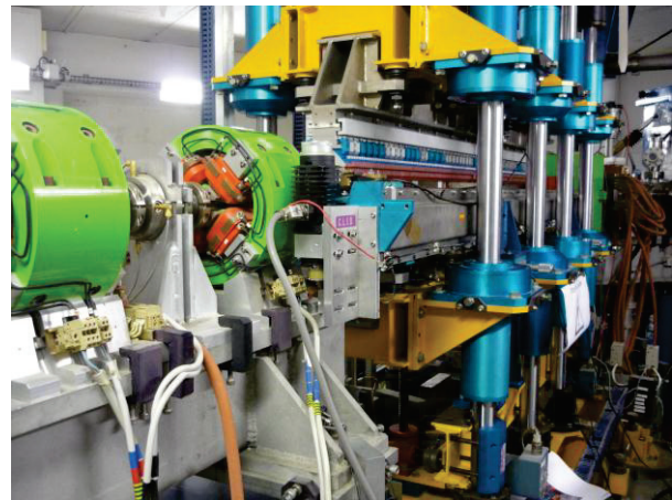
Figure 3: Undulator on-site before mounting the vacuum chamber in order to perform the magnetic measurement. The Hall probe displacement is made by the motor temporarily mounted on the right of the last quadrupole.
