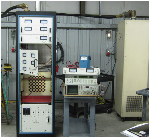
Figure 5: Photo of the whole RF power supply during performance testing.
