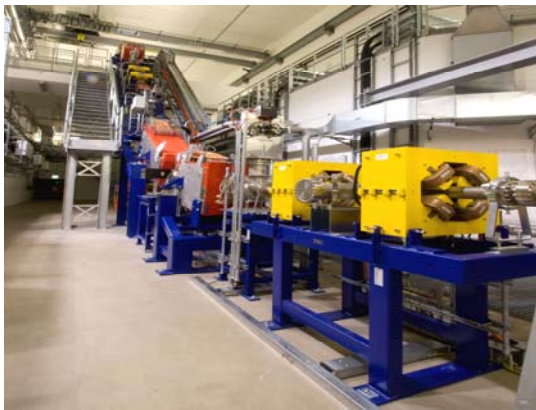
Figure 4: Part of the semi-vertical beam line in the HEBT in Marburg.
