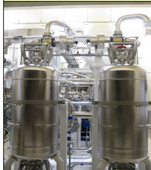
Tritium Processing System
