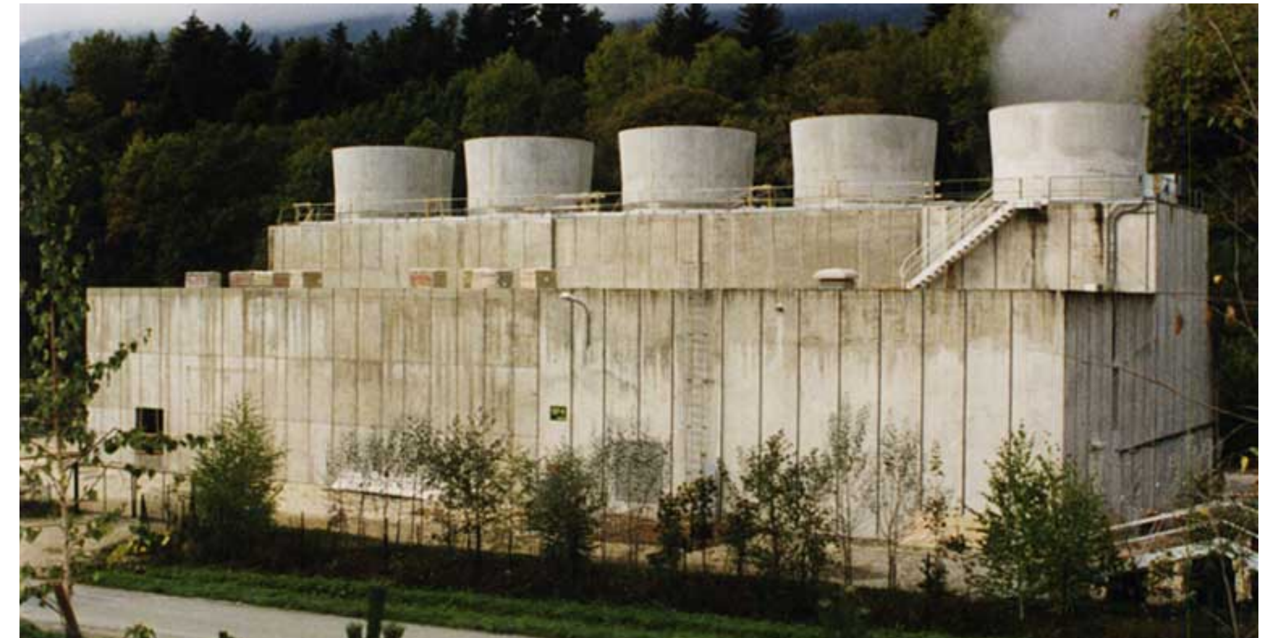
SF4: Cooling tower of LHC point 4
