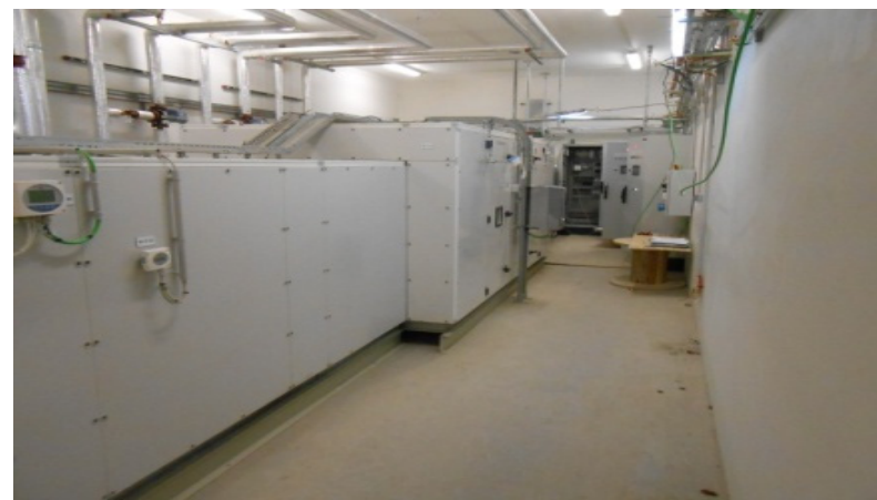
Air Treatment Facility (CTA)
