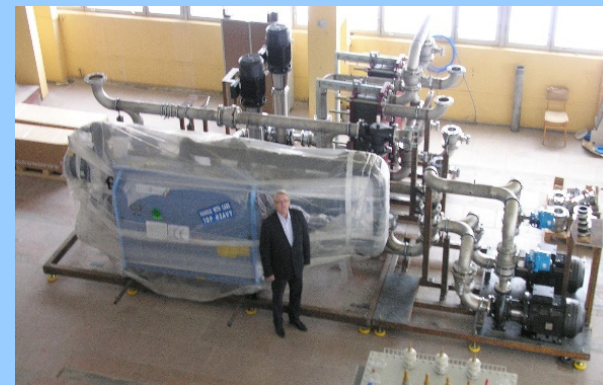
Water cooling system
