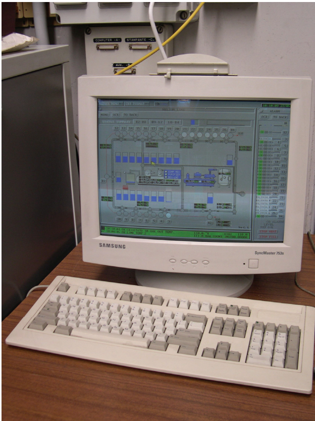
Figure 5: The master PC for the Cryogenics Distribution System.
