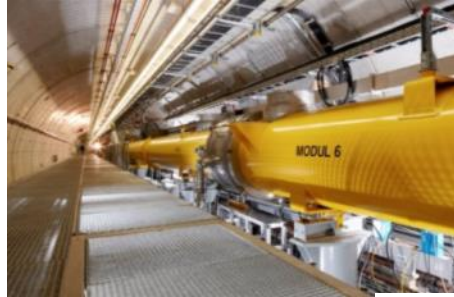
> TESLA type superconducting accelerating modules 1.3 GHz
