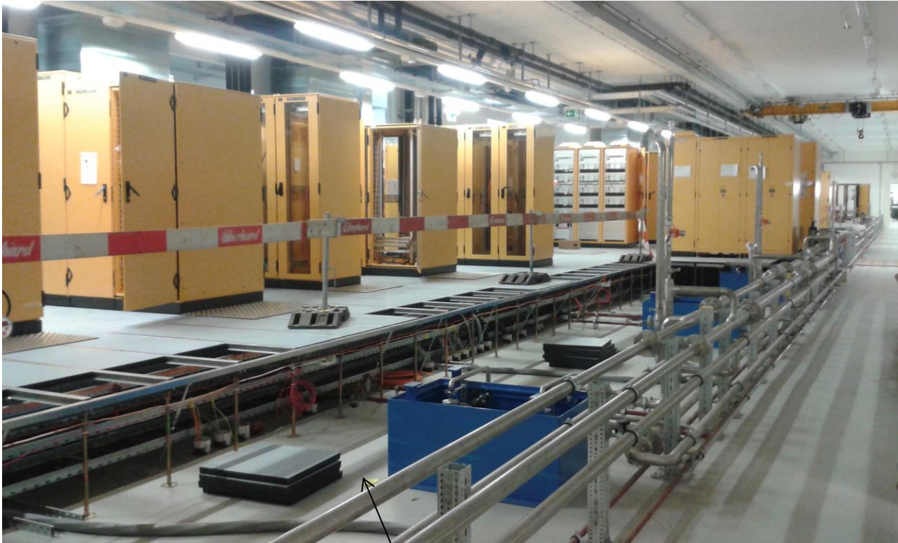
Rack gallery above injector
