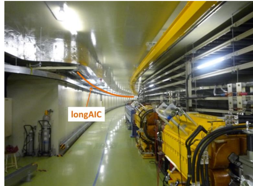
longAIC installed on the cable rack 3 m from the beam line
