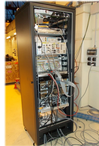
Control and security rack (with fast interlocks)
