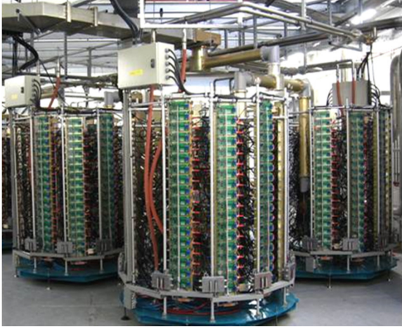
Figure 2: one of the four SOLEIL SR 180 kW SSPA.
