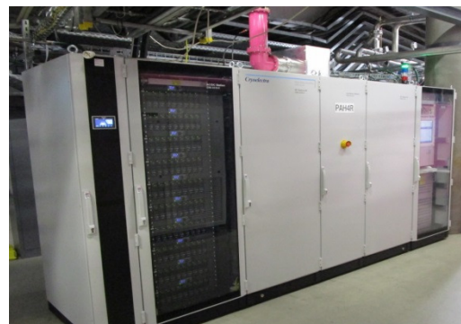
Figure 6: BESSY II 500 MHz 75 kW SSPA.
