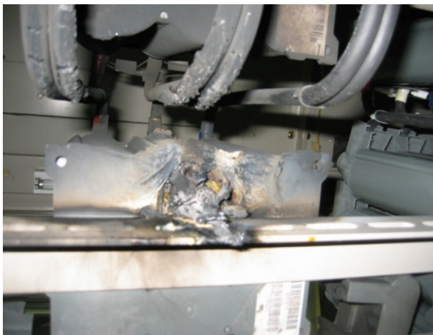
Figure 1: An arc-flash accident took place in the capacitor bank for TLS.
