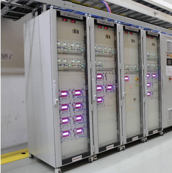
Figure 6: PAL-XFEL magnet power supplies at site.
