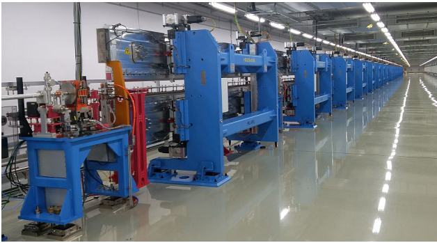
Figure 2: Undulators installed in the tunnel.
