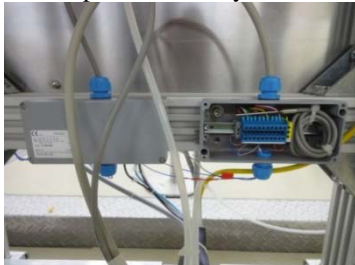
Figure 3: Junction Box with a PT100 sensor.
