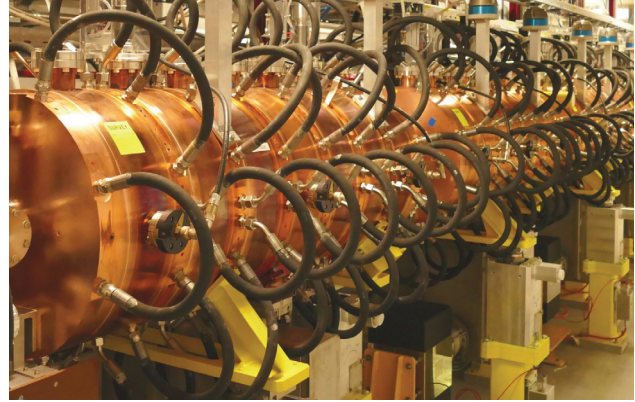
Figure 1: PIMS cavities installed in the Linac4 tunnel.
