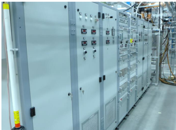
Figure 3: 400 kW DB Science RF Power Station.
