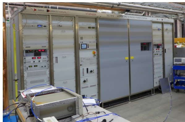
Figure 1: 400 kW Itelco-Electrosys RF Power Station.
