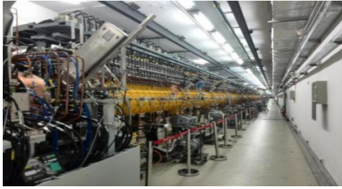
Figure 9: Four tanks of CSNS DTL installed in tunnel.
