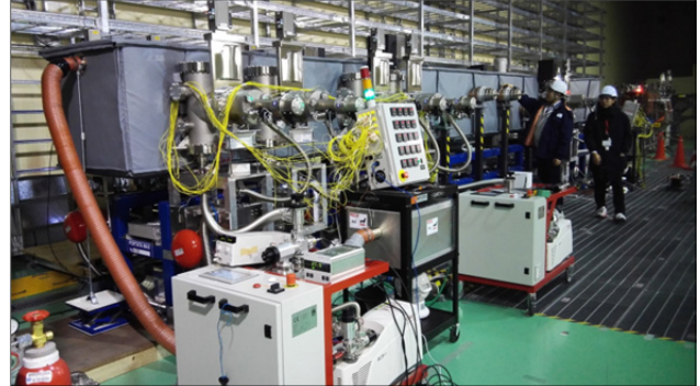
Figure 4: RFQ under baking.
