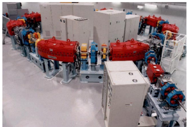
Fig. 10: A multi-purpose synchrotron ring at Wakasa-Wan Energy Research Center.
