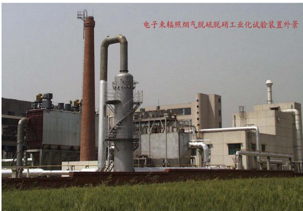
Figure 8: pilot plant constructed by CAEP for removing SO 2 and NO x in Mianyang, Sichuan
