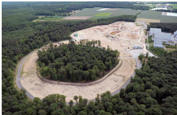
Figure 2: Aerial photo of the construction site taken on May 25, 2014 (photo: J. Schäfer, FAIR).
