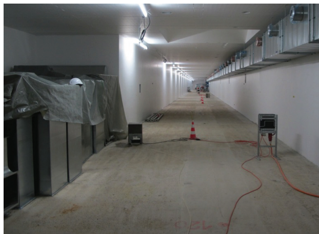
Figure 7: Picture of the empty SwissFEL accelerator tunnel.
