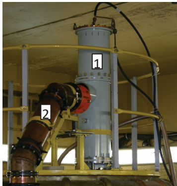
Figure 3: External view of UPI: 1 – UPI; 2 – channel of HF power transfer.
