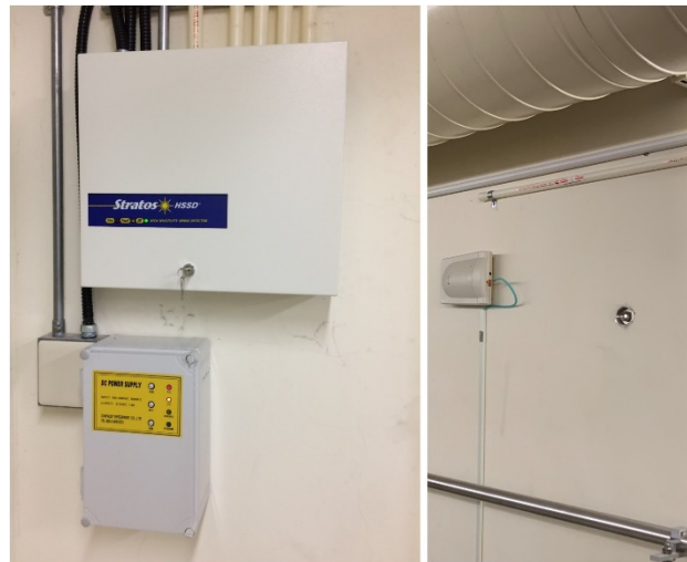
Figure 7: Aspirating smoke detector installed in the CIA room outside of the tunnel (left) and sampling pipes in the tunnel (right).
