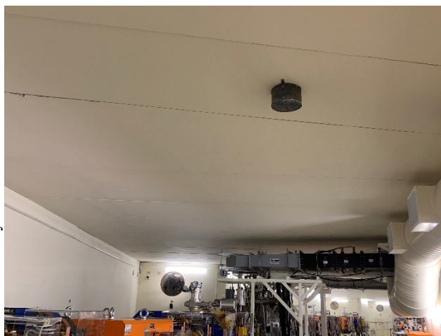
Figure 6: Smoke detector with lead shielding.
