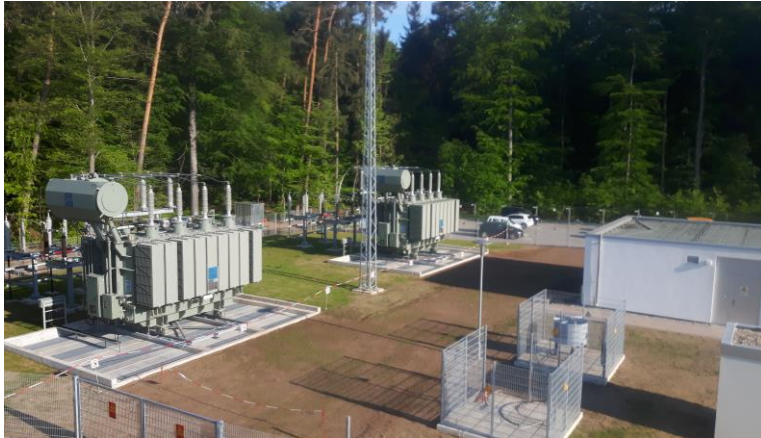
New transformer station North completed. (pulse power SIS18 and SIS100).
