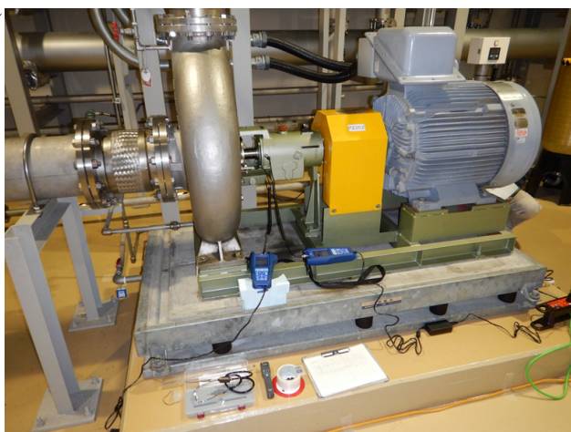
Figure 1: Circulation pump P2202.
