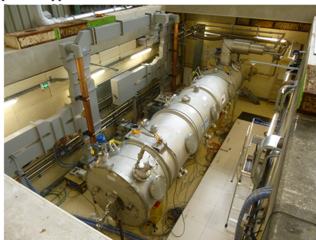
Figure 1: M-ECCTD cryomodule installed in the test station at CEA (with roof removed).
