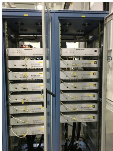
Figure 4: Pictures of processor hardware and cabinet.
