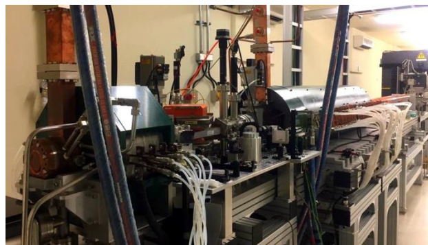
Figure 4: The NSRRC photoinjector in the ATA tunnel.
