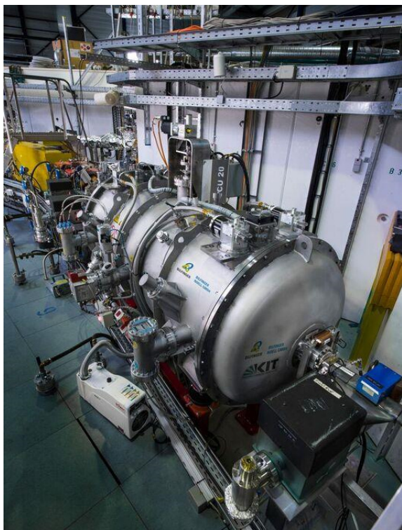
Figure 1: SCU20 installed in the storage ring KARA of the KIT synchrotron.
